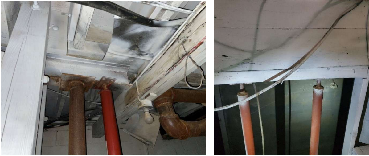
Figure 39 & 40: Pipe Jack Supports in Basement Level
