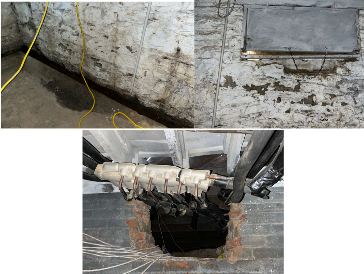
Figure 14: Examples of water infiltration and related damage in the basement/foundation walls.
