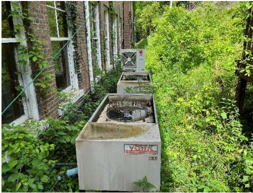
Figure 59 - Condensing unit on ground.
