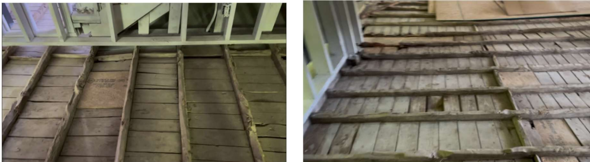
Figures 20 & 21: First Floor - Main Hall Rear of Entry – Damaged Floor Joists
