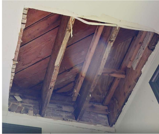
Figure 33: Second Floor Ceiling Cutout Revealing Third Floor Framing Above
