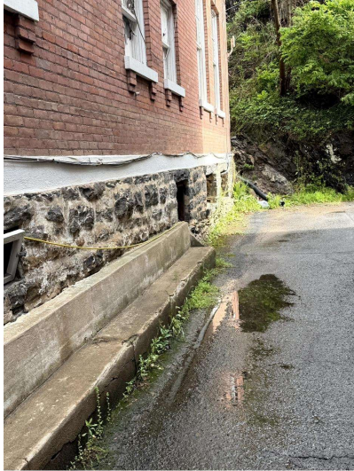
Figure 5: view of the east-side access drive showing pavement deterioration, ponding along the foundation interface, vegetation encroachment, and lack of positive drainage. A basement window / vent opening is visible at grade in the stone foundation wall.
