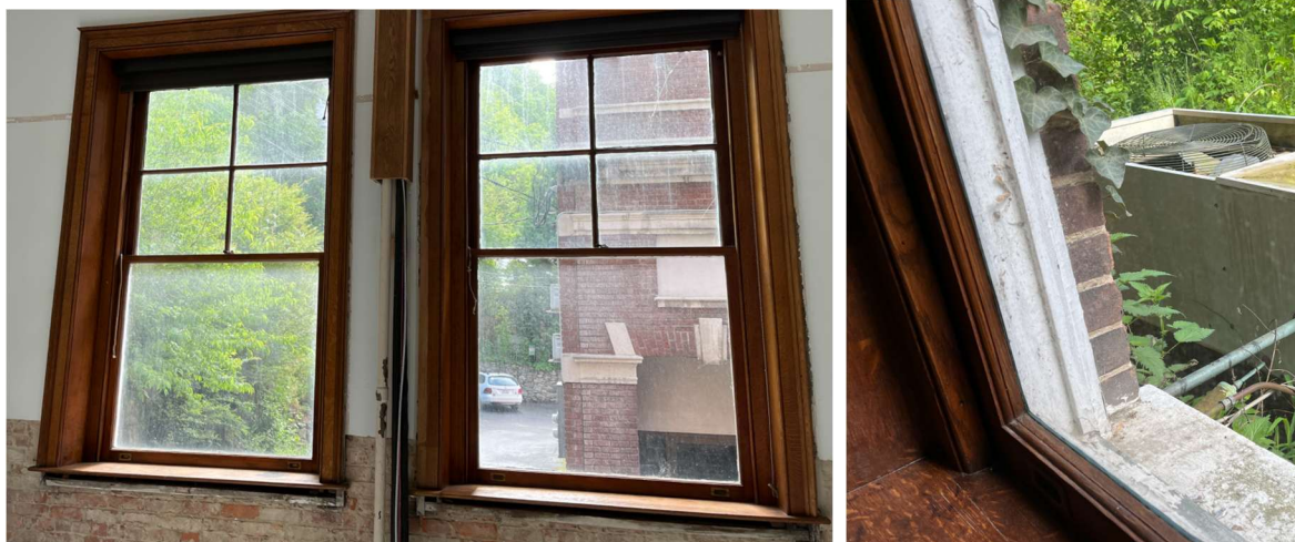
Figure 13: Example of existing single pane windows to be replaced.
