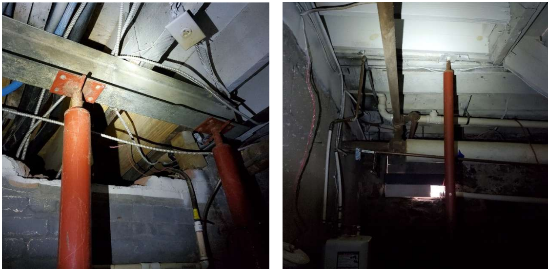
Figure 41 & 42: Pipe Jack Supports in Basement Level
