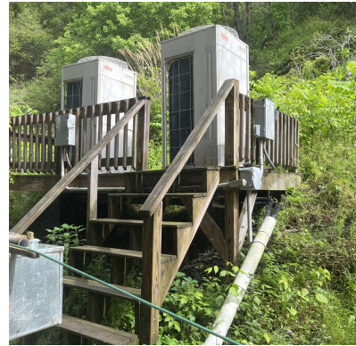
Figure 60 - Multizone Heat Pumps
