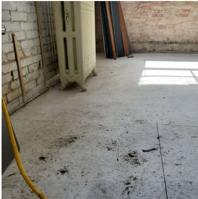
Figure 27: First Floor - Rear East Room – Low Spot in Subfloor at Radiator Heater
