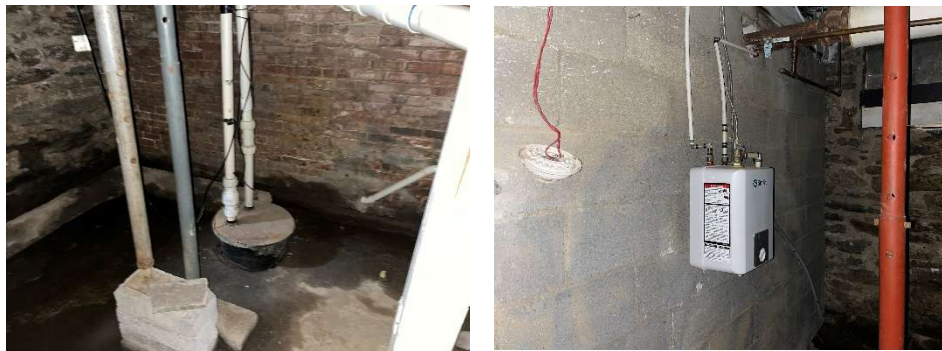
Basement sump pump and wall mounted instantaneous water heater.
