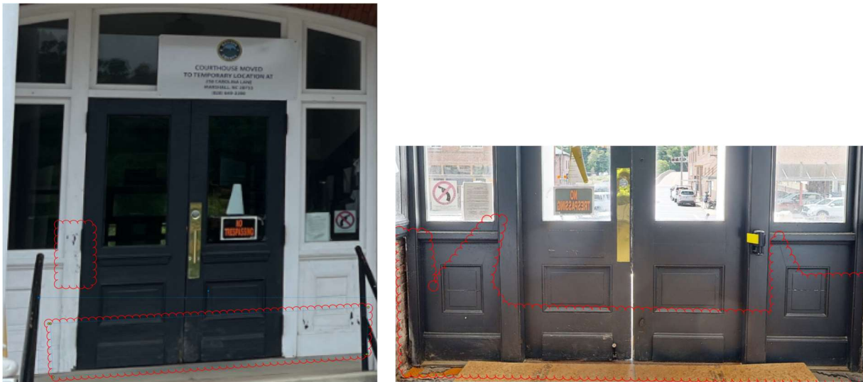
Figure 7: Photos of the original main entrance doors with special attention to visible water damage including rotten wood on the doors and framing elements, visible fissures in wood panels, large gaps, and rotten subfloor elements.
